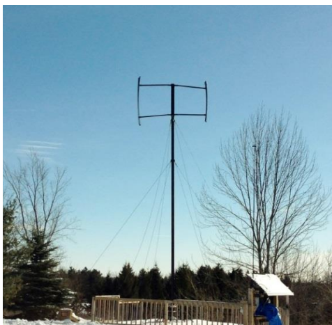
FireflyPower field installation at Oak Ridges Moraine
